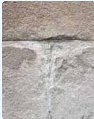
Deterioration of block corners.
