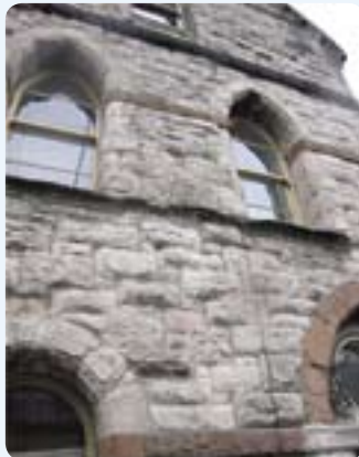
Widespread surface deterioration of stonework with loss of architectural detail.
